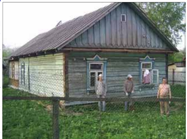
Three members of Ratomka Bible Baptist Church help Sergei dismantle this log house we bought for $1000! The logs and materials are being used to build the Virtual Orphanage Foster Home this summer.
