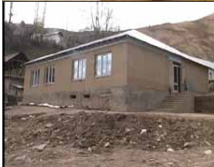
Above shows the roof we built on the school in Pishanbye last September. This school is near Poshum where we are building a school this year.
