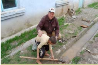
Above –We cleaned a ton of garbage out of the Soviet built water storage tank. Orphans earned a paycheck helping sift and wash sand for masonry work in the orphanage shower and laundry facilities.
